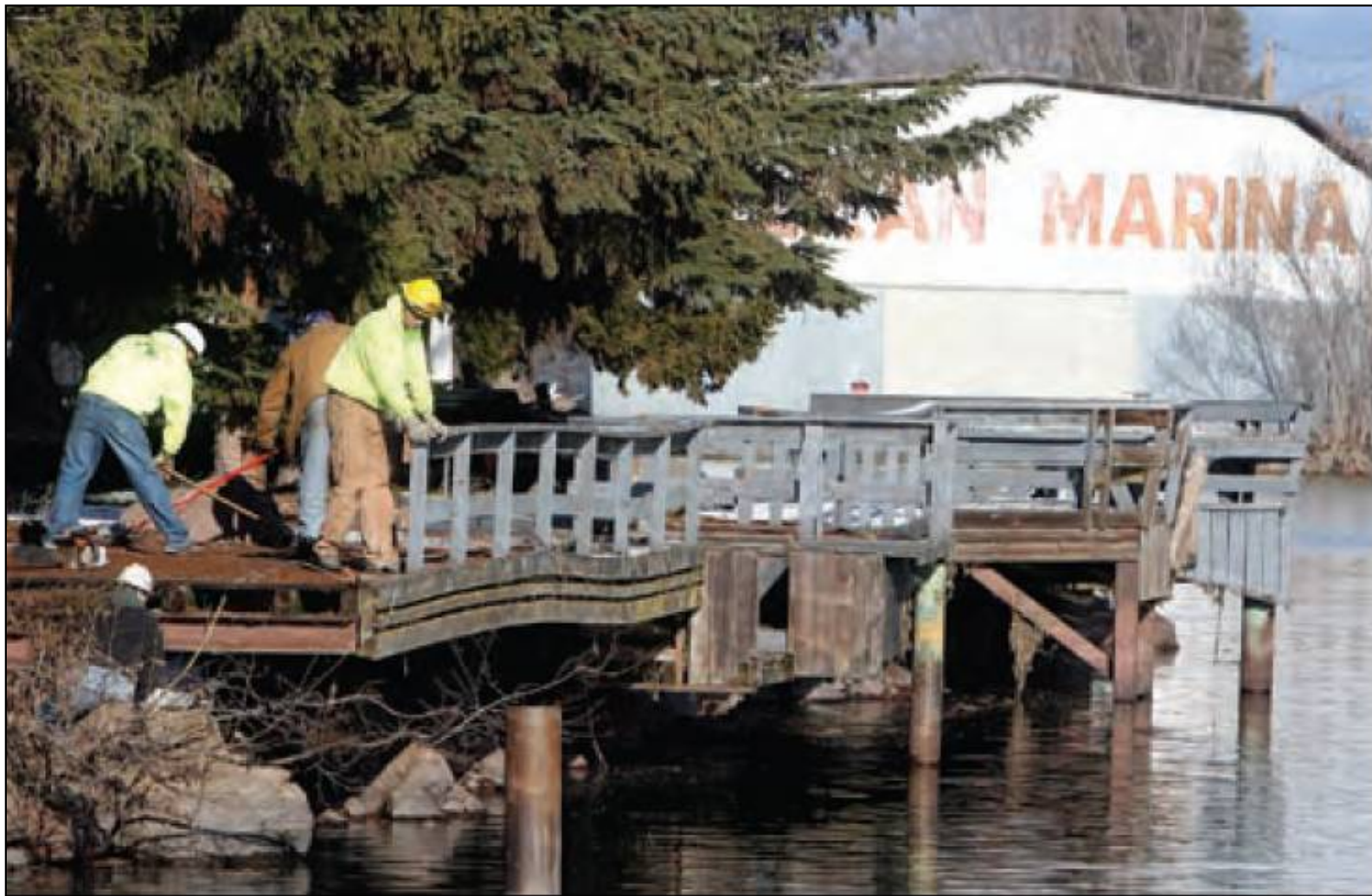
A crew from Rocky Mountain Construction demolishes the landing at Putnam's Point Park Thursday. Work on a new pier should start this summer.
