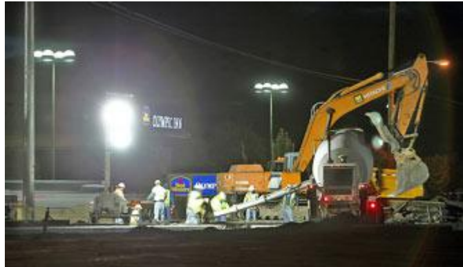
H&N photo by Andrew Mariman Concrete is poured at the intersection of Washburn Way and South Sixth Street.
