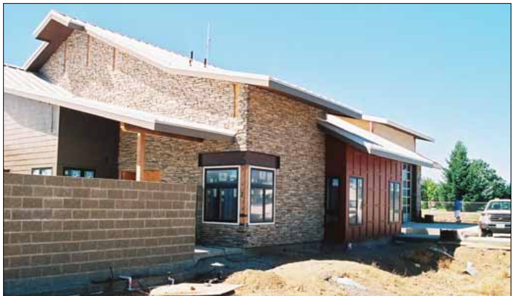
The Redwood Substation is designed to blend into the residential neighborhood.
