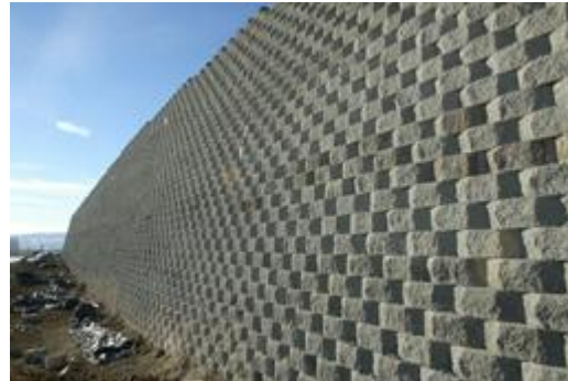
The retaining wall at the new Herald and News building site measures 650 feet long and contains about 12,000 cement blocks filled with gravel.
